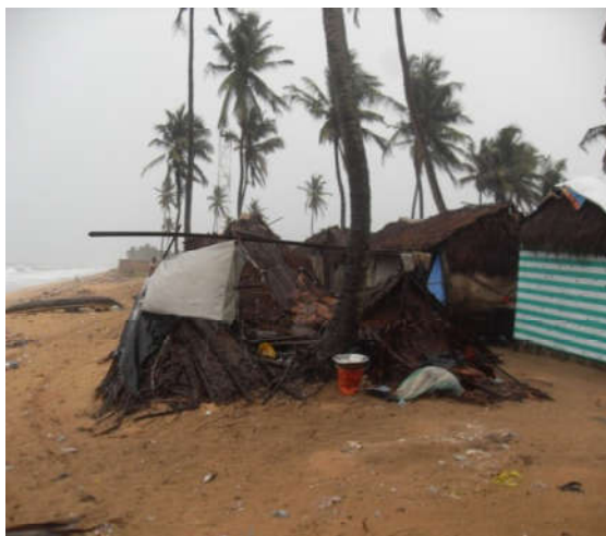
Plate 13: A destroyed house at Pengbo
